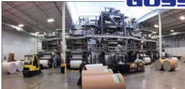
The completed installation of the first triple-wide Goss Uniliner press in the USA.
